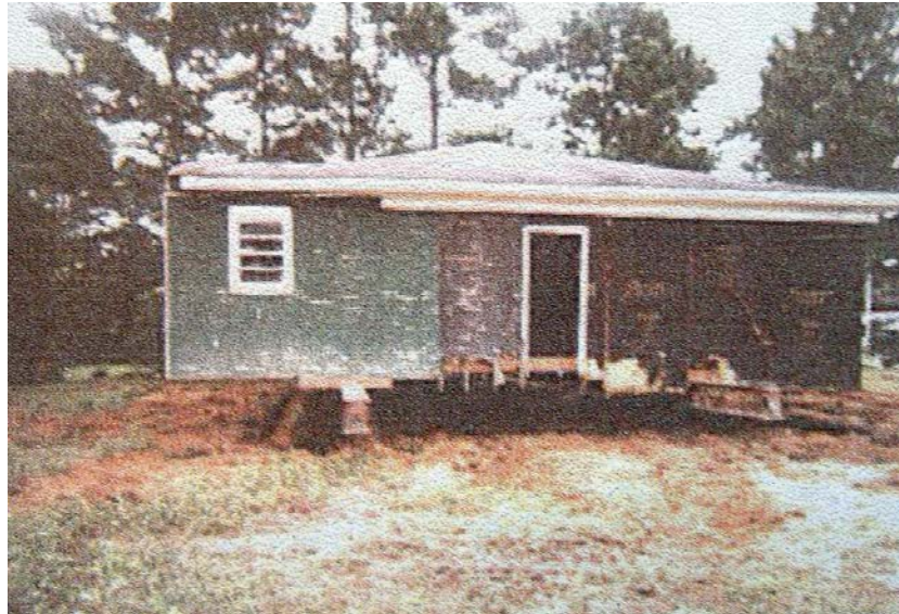
Figure 2: State of one of the two flooded homes that ended up next to the Johnsons house, before refurbishing, summer 2001. Source: William Johnson.
